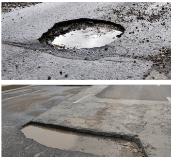
Fig. 7. Example of potholes.
